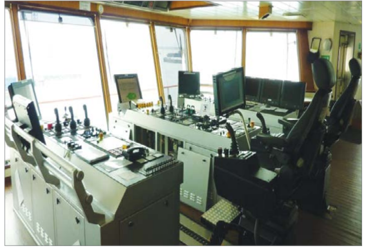
Rear facing bridge control
